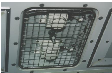
Smoke detector / fire extinguisher nozzle panel on the ceiling of the cargo hold
