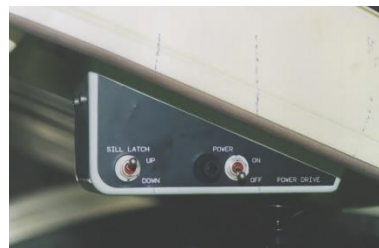
ULD movements in compartments are controlled with the joystick. The power ON-OFF switch of the cargo loading system and sill latch UP-DOWN switch are located on the right hand side of the joystick assembly.
