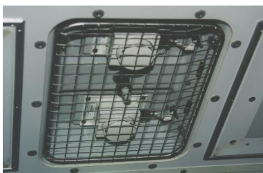
Smoke detector / fire extinguisher nozzle panel on the ceiling of the cargo hold
